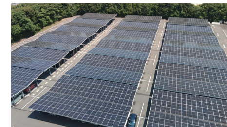
Installation of Solar Panels in the Parking Lot at the Shiga-Yasu Plant
