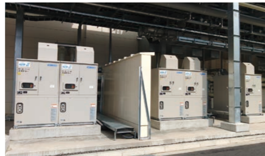
Kyoto Ayabe Plant: Exhaust heat recovery
