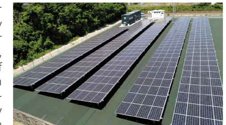
Yasu Kamiya Solar Power Plant (Solar power generating system and stationary lithium-ion storage battery)
