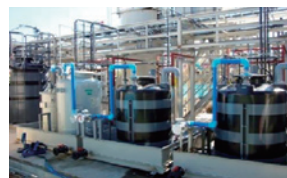
Chemical processing facility for polluted groundwater
