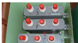
PCB storage box (Shiga Gamo Plant)
