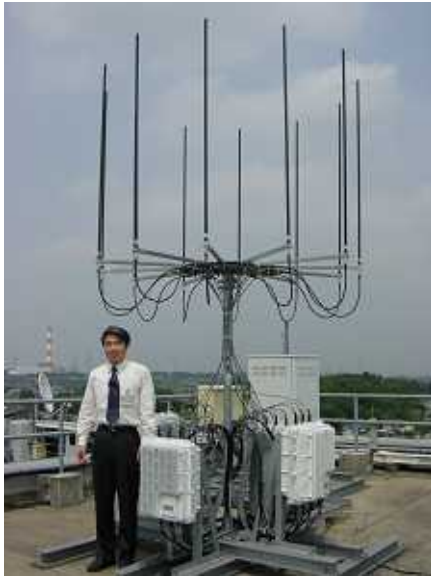
Fig. 1: iBurst Base Station
