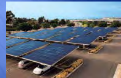
Installation ex; Parking lot
