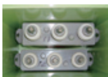
PCB storage box (Shiga Gamo Plant)
