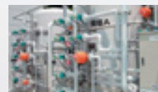
Ion exchange tower
