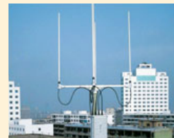
G3 base station
